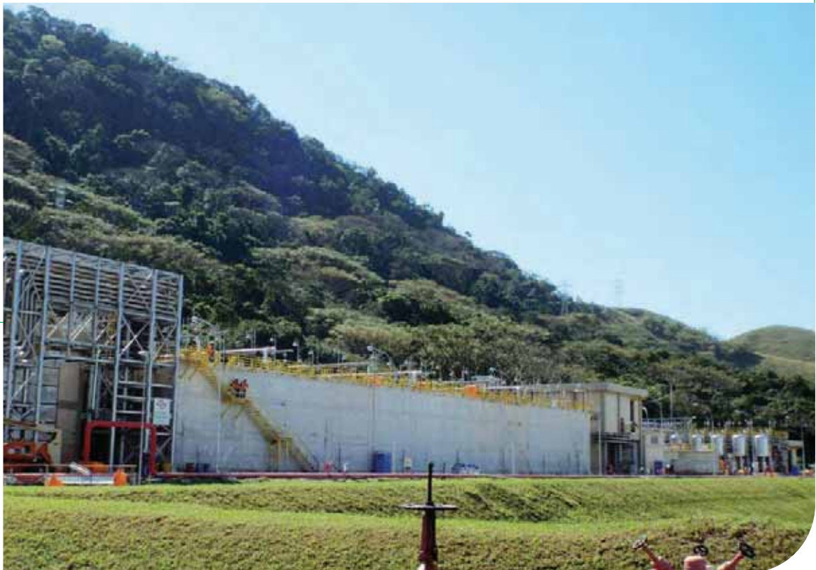
Effluent Treatment Station at Almirante Barroso Terminal (TEBAR), São Sebastião (SP)
